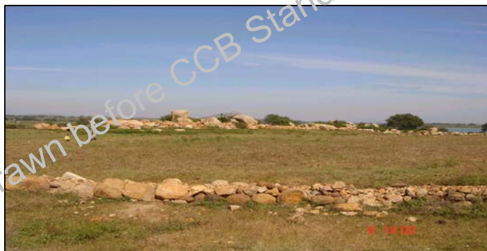
Fig B-1: Dry land development work in the proposed A/R CDM project area
